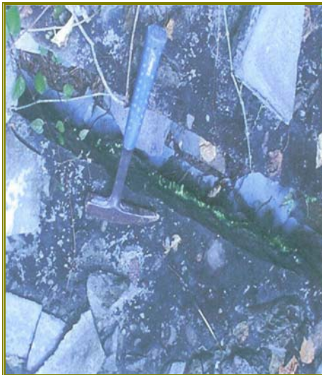
Photo 16 Crack opening in foundation of house
