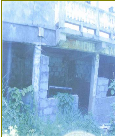
Photo 15 Evidence of movement in one of the houses at Gibson
